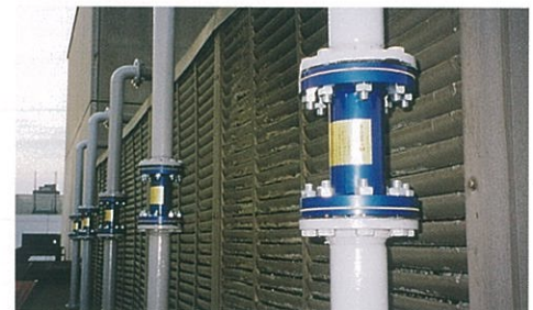
Treatment of sprinkling water in a closed cooling tower
